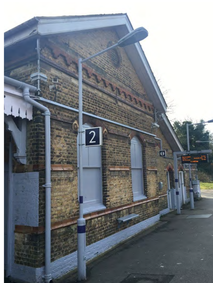
Plate 10: Boarded windows to the platform elevation
