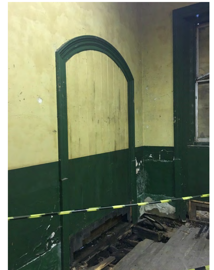
Plate 23: Boarded up door within the 'Booking Office'
